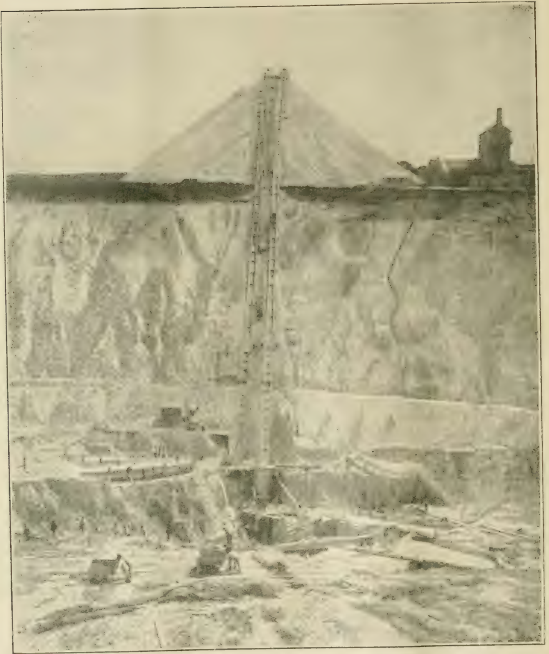
FIG. 4 DOUBLE INCLINE AT THE BOTTOM OF A DLET PIT WHICH IS BEING WORKED IN TWO STAGES.
